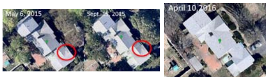
Shingles seen shifting and lifting from the roof after the Winter Storm Event
