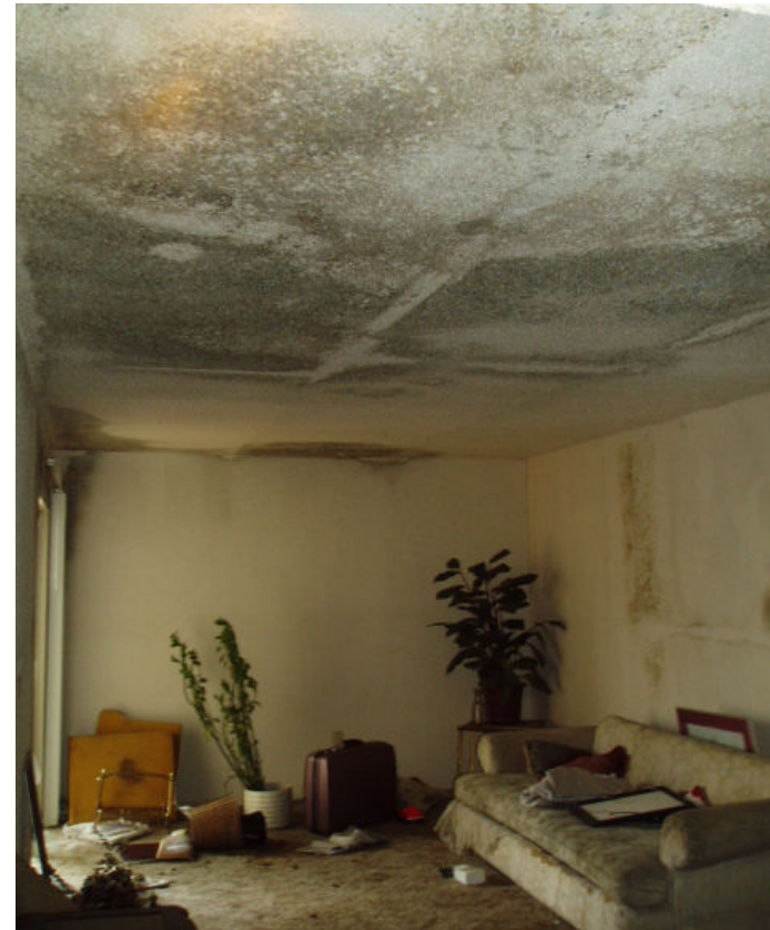
Evacuation left water penetration unattended for two weeks in summer heat and humidity
