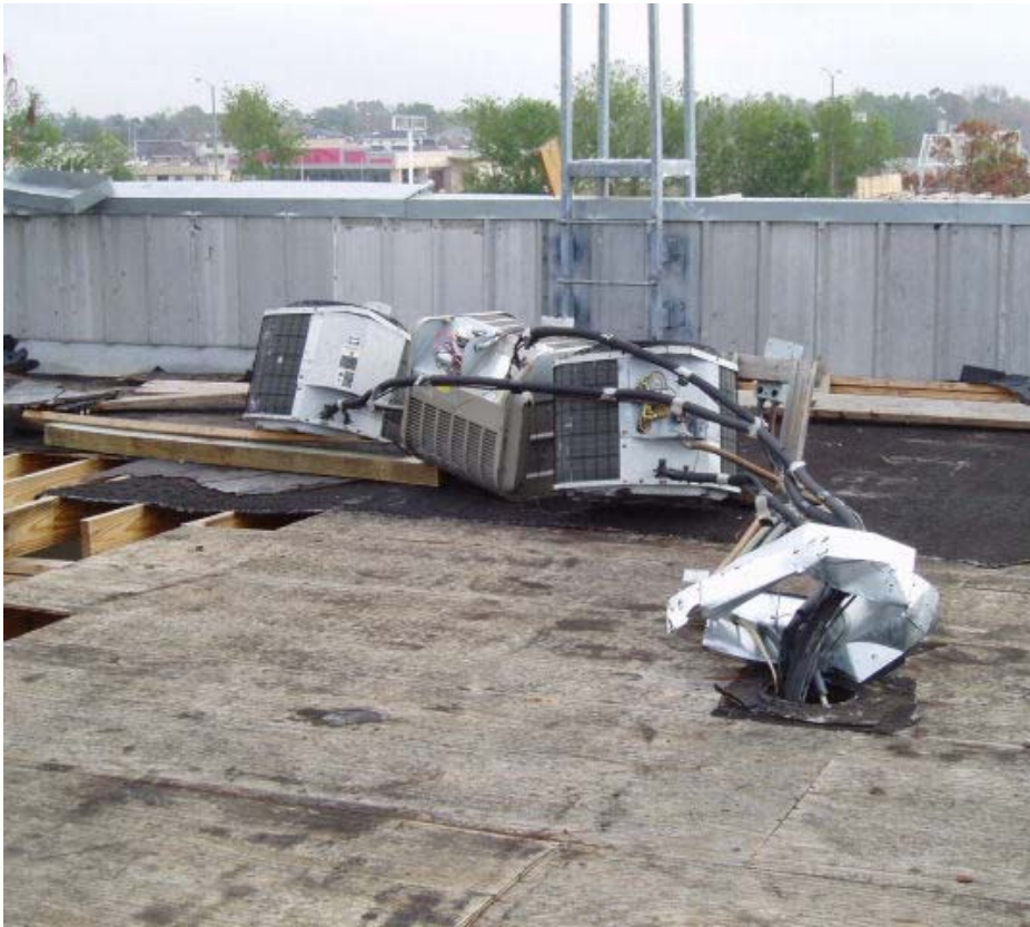
Roof damage and air conditioner ducts torn open, lets rain penetrate through 1 ft duct
