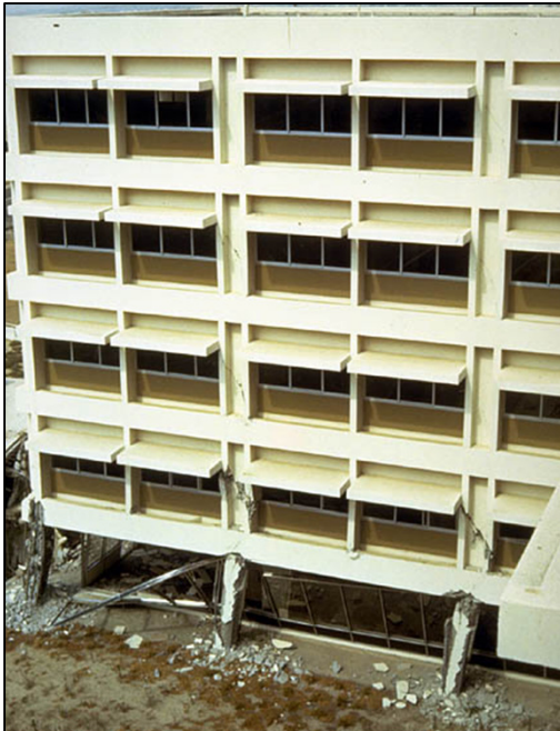
1971 M6.6 San Fernando Earthquake
