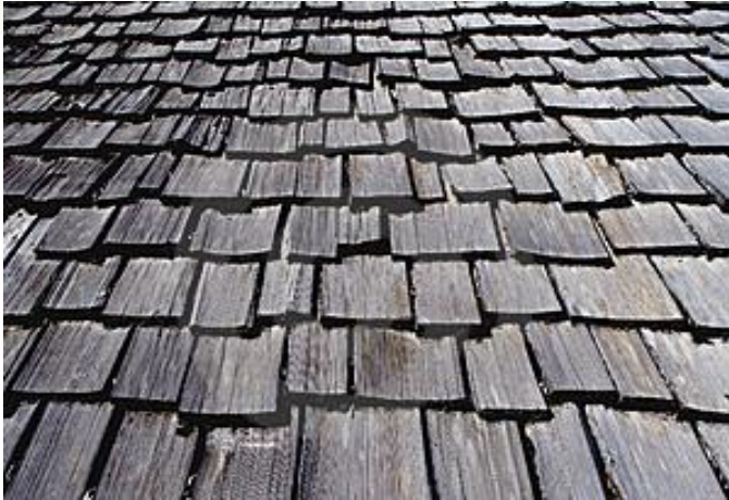
Wood shingle roofs are extremely vulnerable
