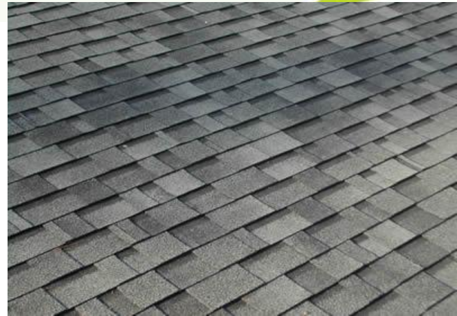
New asphalt shingles are excellent, but decompose with time
