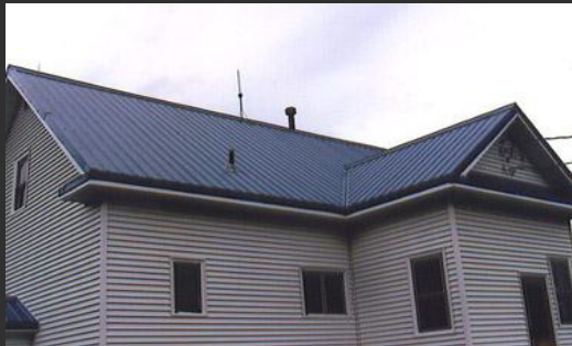
Original Inspection Findings
